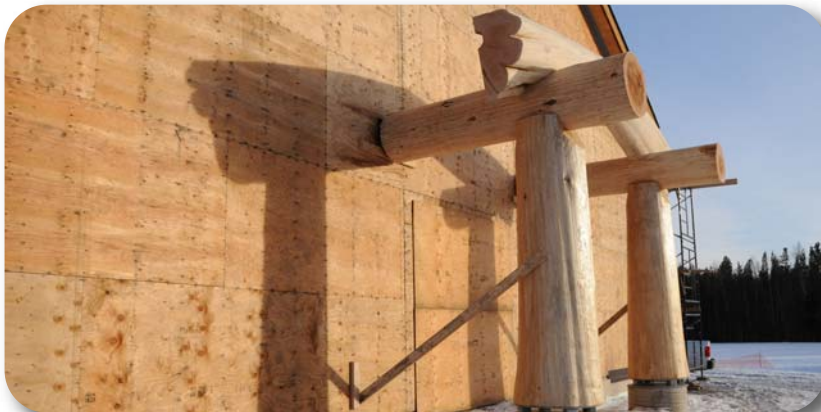
Work progresses on the Longhouse. Seen here is the western entrance catching the winter sun. For more, visit the photo gallery on the NWCC HomePage.
